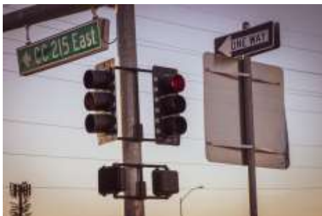
Central Traffic System Upgrade
